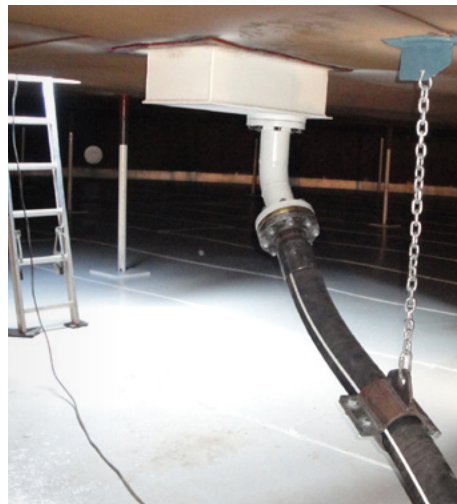
CTS tank drain hose at centre sump.
