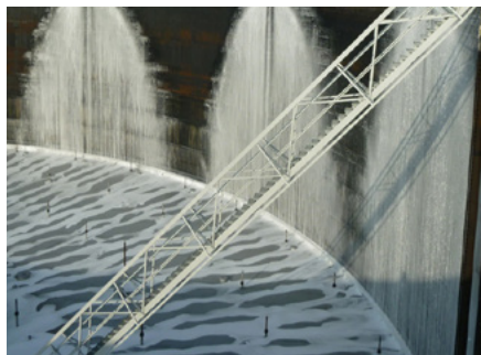
Live foam test on external floating roof tank with an integral foam dam.
