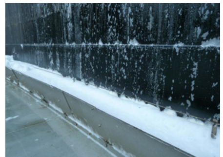
Integral foam dam immediately after live foam test.
