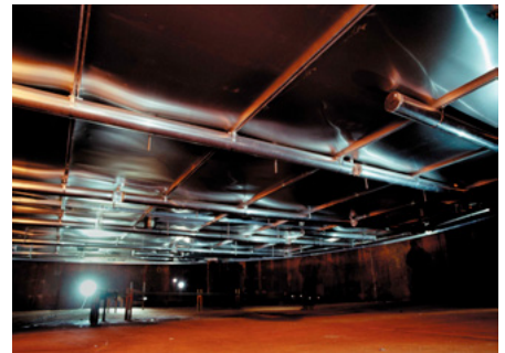
Cable suspended skin and pontoon IFR, bottom view.
