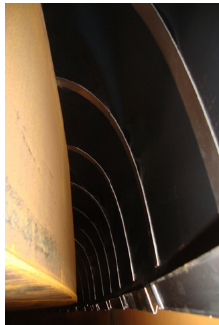
CTS30 primary seal on steel floating roof.
